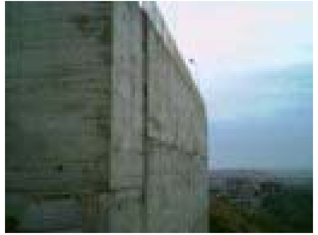
Fig. 2. Picture of failing wall type 30.
