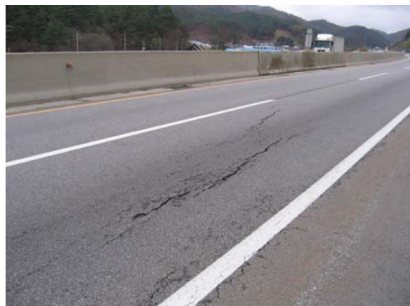
Pic.8 Cracks of the eastbound lane pavement
