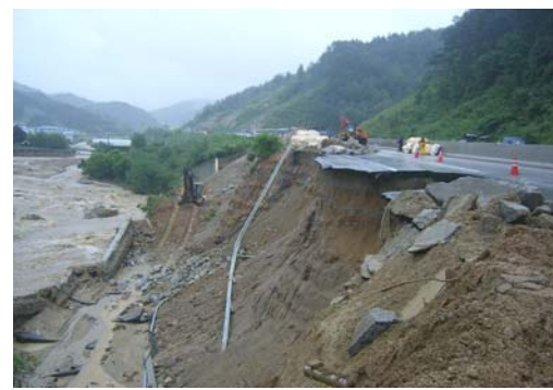
Pic.1 Destroyed embankment
