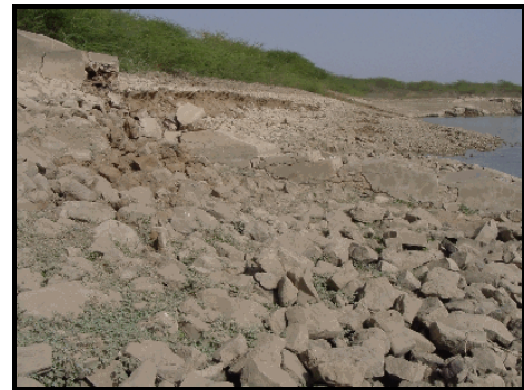
Figure 1h: Cracking and Slumping in the upstream face of Rudramatha Dam
