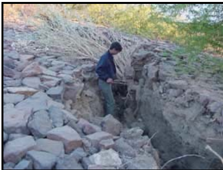
Figure 1e: Massive cracks in the upstream embankment near the toe of the Fatehgarh dam
