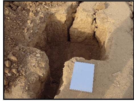
Figure 1f: Longitudinal cracks in the crest of Kaswati Dam
