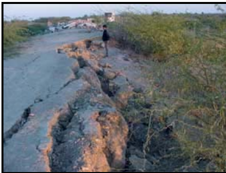
Figure 1d: Upstream slope failure of Fategarh Dam
