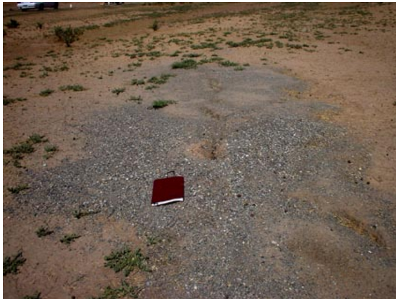
Figure 3. Liquefied gravel at point B
