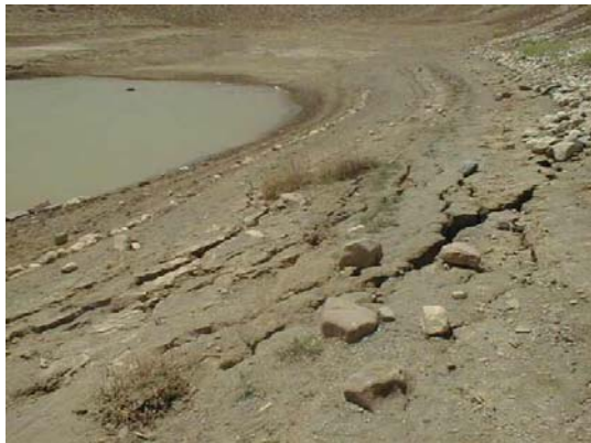
Figure 9. Instabilities at upstream slope from a closer view
