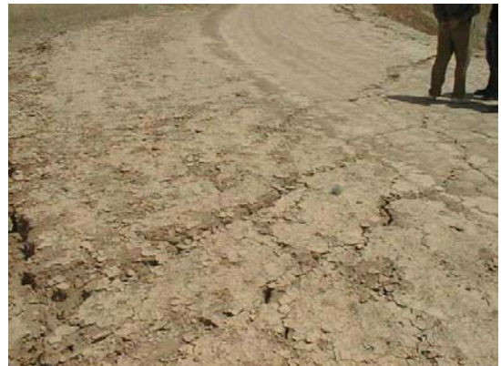
Figure 10. Cracks crossing the body of dam at its left abutment
