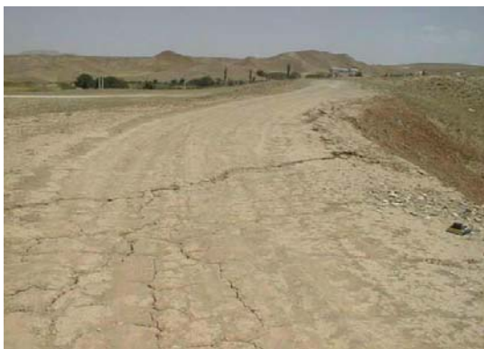
Figure 11. Cracks crossing the body of dam at its left abutment
