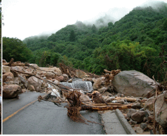
Fig 18. Loss of road example
