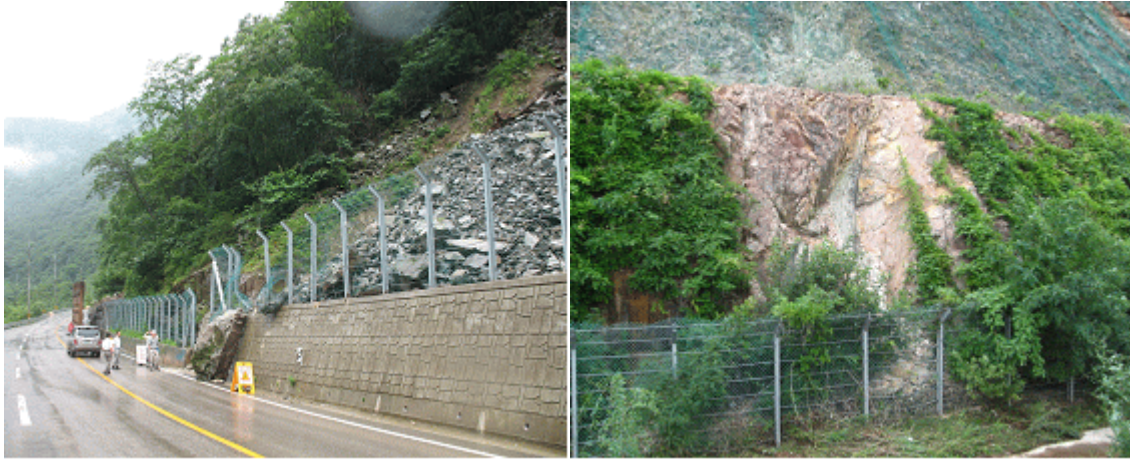
Fig 4. The Damage Example due to Stone falling
