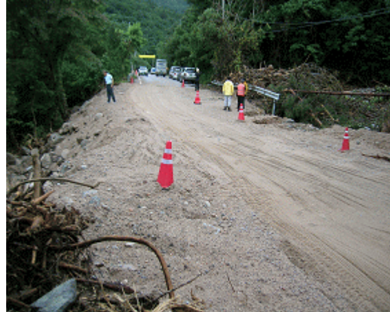
Fig 14. Damage to a road due to overflowing water
