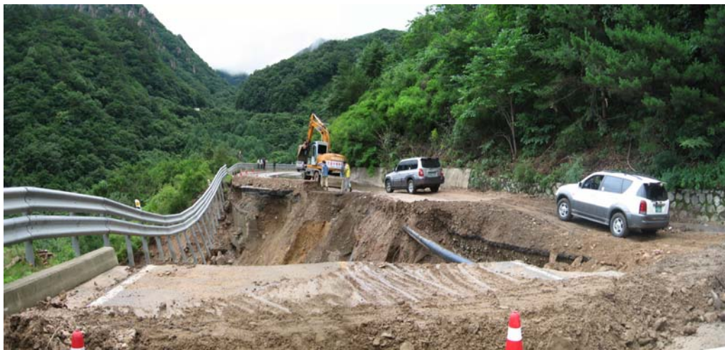
Fig 9. The damage example by banking section
