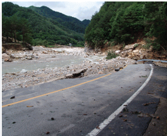
Fig 12. Picture of failure due to water impact
