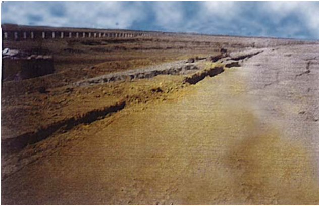
Fig. 4. Longitudinal crack over the length of the embankment
