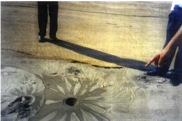
Fig. 5. Wet hole on February 11, 2001 from which water and silt had oozed out
