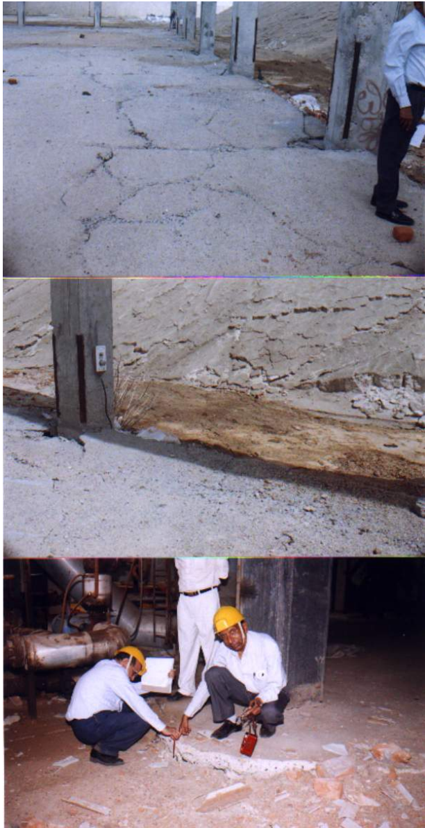
Fig. 9. Settlement of the surrounding flooring and the entire flooring of the stacking go-down is cracked
