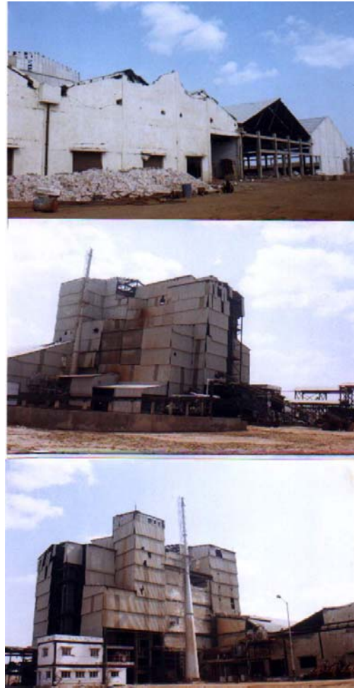
Fig. 8. Structure of salt factory after the earthquake
