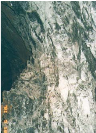
Fig. 3. Side wall scaling in 1571m cross-cut drift
