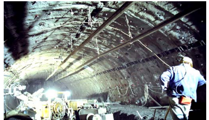
Fig 12. Three rows of yielding elements installed in the shotcrete lining at the Semmering base tunnel
