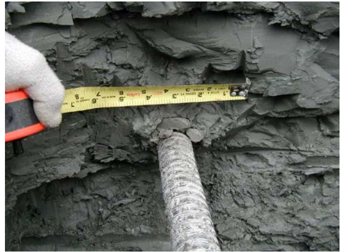
Fig 11. Nail hole annulus. Majority of 6-inch-diameter hole is soil cuttings, with some grout around nail bar
