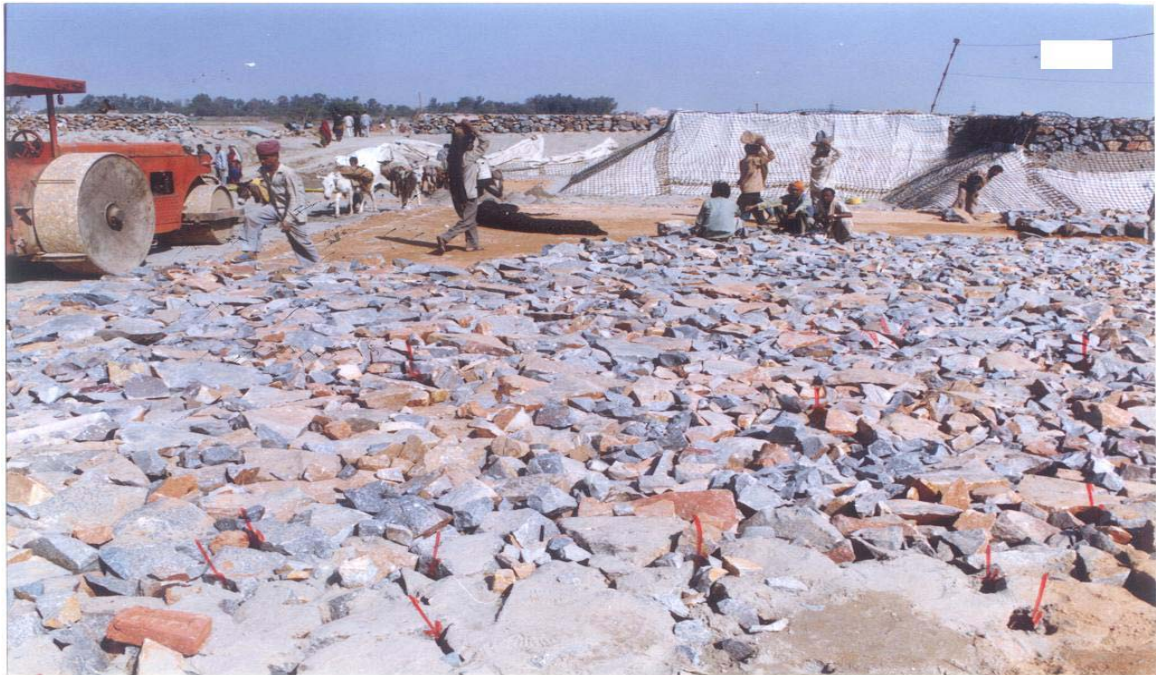
Fig.6(b). Photo plate showing the geo fabric, overlaying rope mattress and stone
