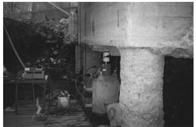
Fig. 11. View of the load test on a pile of the piled foundation.
