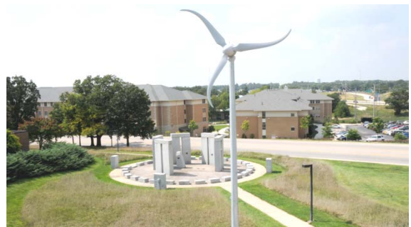
Fig. 1. Skystream wind turbine installed at the authors' university
