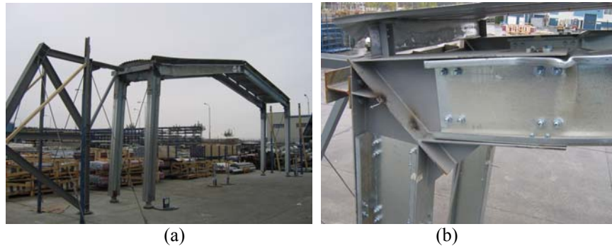
Figure 10. C1 frame: global view (a) and local buckling of the left beam connection (b).
